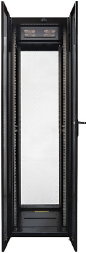
Views of the cabinet without side panels and rear cover:
